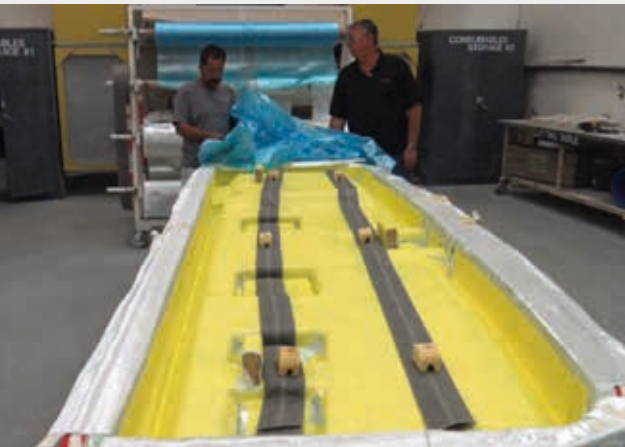
3. 510 Fly swim platform ready for bagging after Compoflex® RF 3 has been installed.
